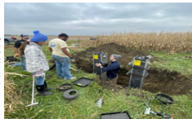
Controlled Drainage (South Dakota site)
